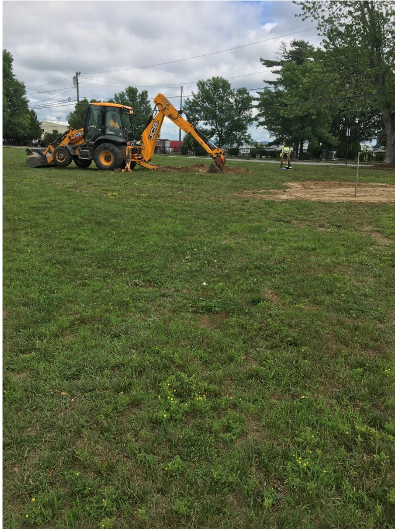
Airport Dr existing site photo drilling test pits (photo provided by the City of South Burlington)
