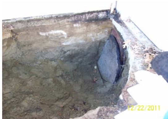
Plate 4 Hole in UST covered before excavation backfilled
