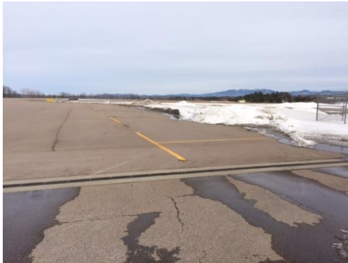
Photograph F-1. Valley West Apron (Facing east from southeast corner of Apron)
