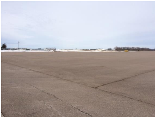
Photograph F-3 Valley West Apron (Facing northeast from south end of Apron)
